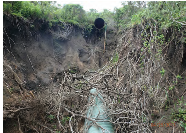
Damaged drainpipe causing gully erosion
