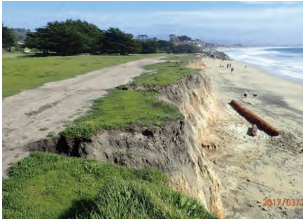
Eroding trail at the Mirada Surf West (Coast)
