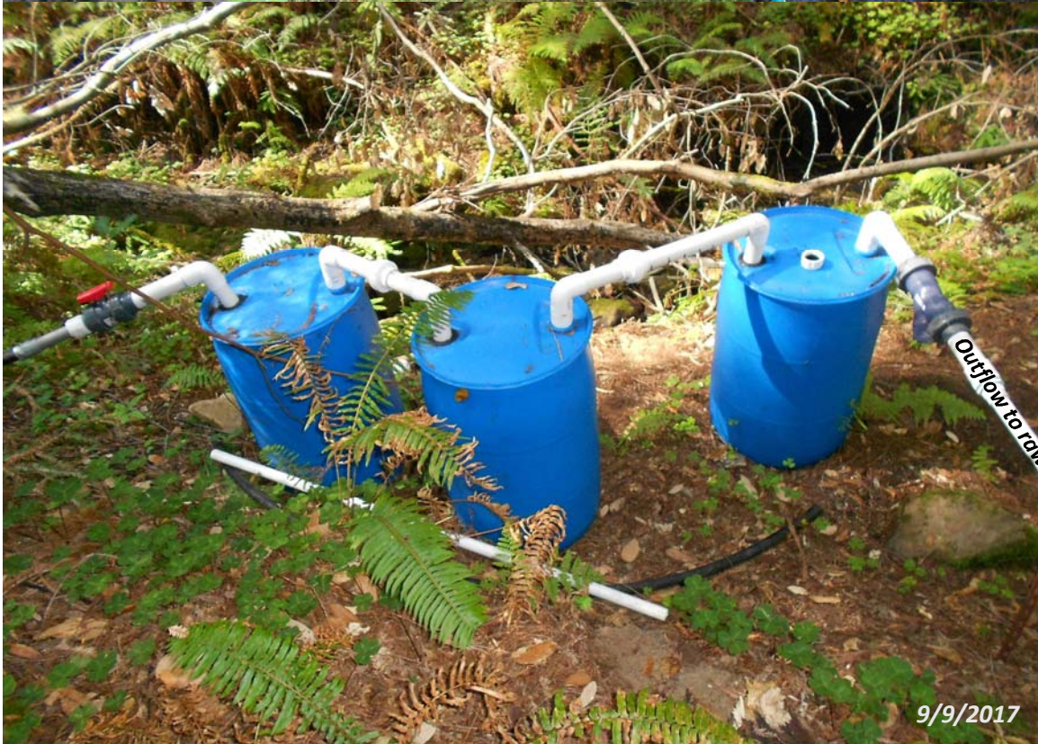
Figure 1. Existing diversion structure on Hoffman Creek, Redwood Glen, San Mateo County, CA. The diversion structure consists of a stainless-steel sink attached to a redwood log across this creek. Sediment entrained in the line extending from the sink to the raw-water tank accumulates in a series of three 55-gallon drums used for settling. Water and sediment is flushed onto the bank during maintenance twice a year.
