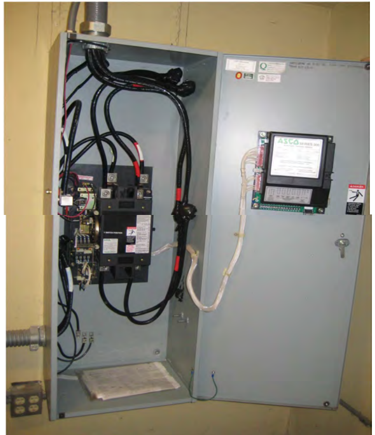
EE3 – Automatic transfer switch
