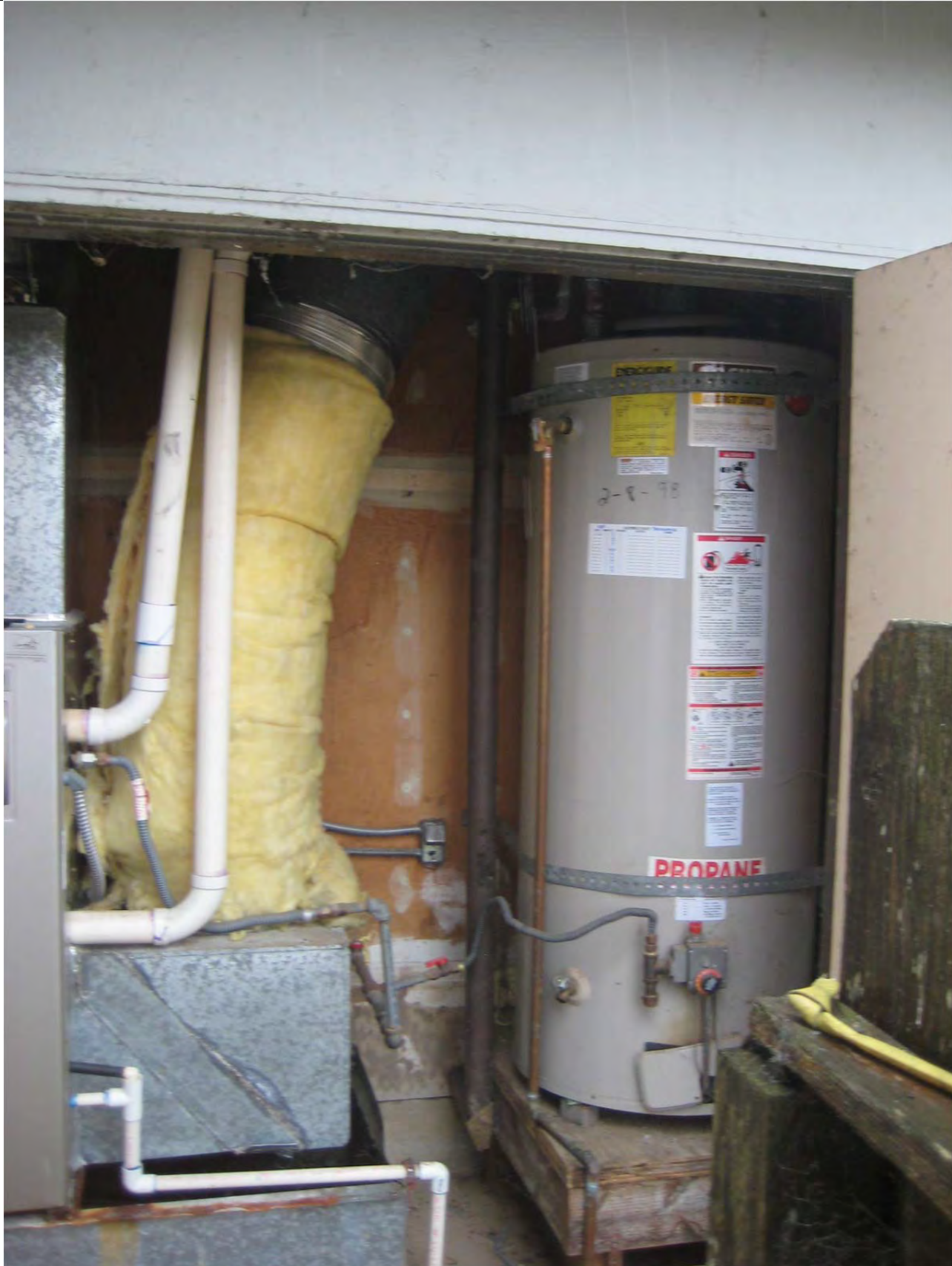
ME1 – Water heater and furnace
