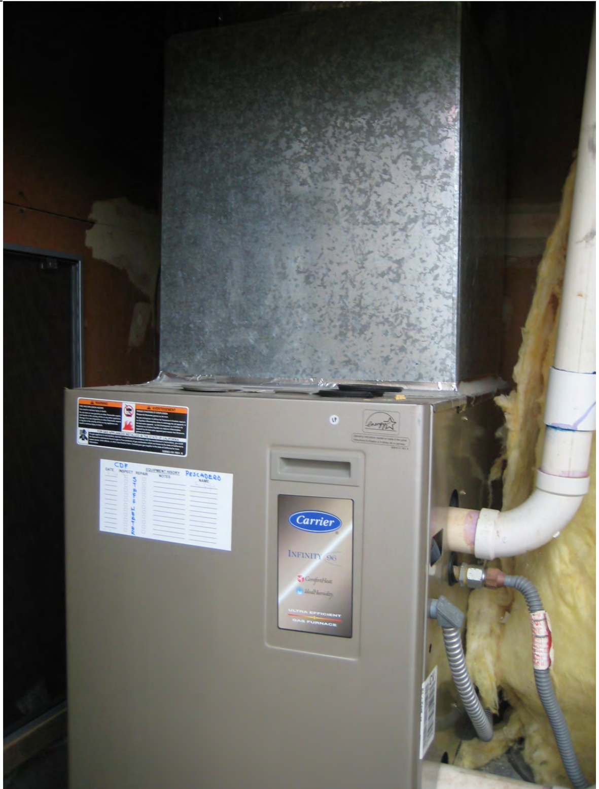
ME2 – Gas furnace
