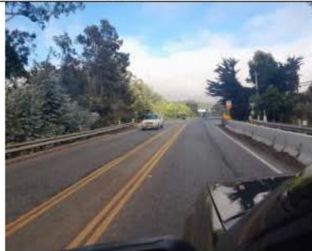
Photo 6: SR-1 at Medio Creek is very dangerous to cross so the culvert underneath the roadway has been used for decades by residents of Miramar.
