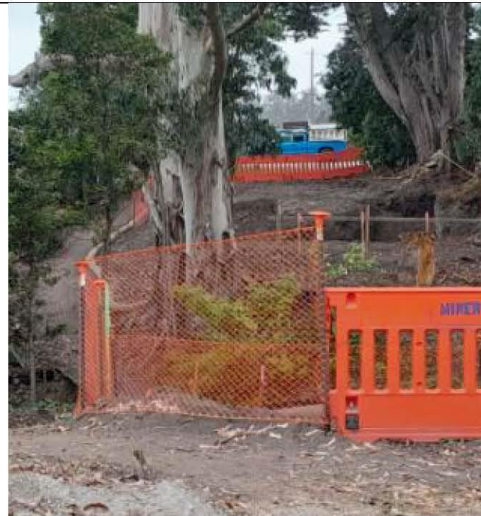
Photo 4: Examples of current construction at Medio Creek where excavation occurred directly adjacent a large eucalyptus impacting the shallow root system.
