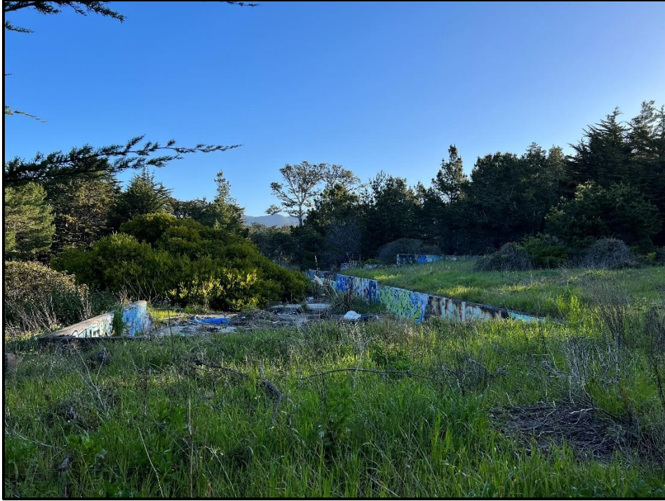
Photo G-5. View facing north showing the remnants of concrete foundations situated in the northern portion of the BSA. Photo taken April 4, 2023.
