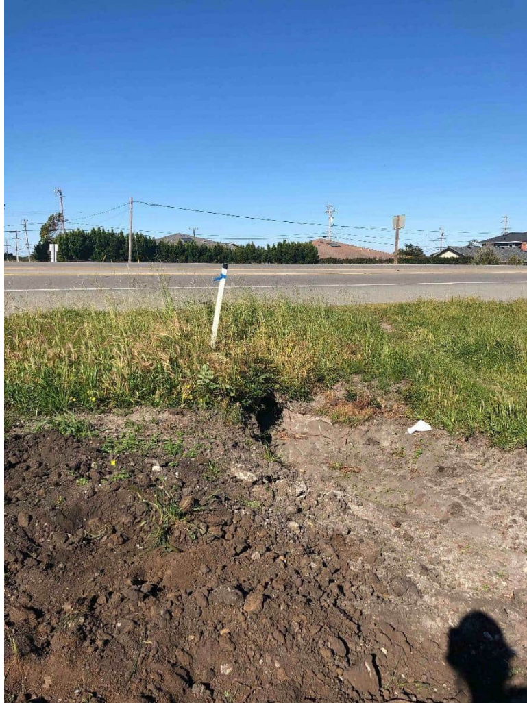
Photo 2. View of eroding culvert.
